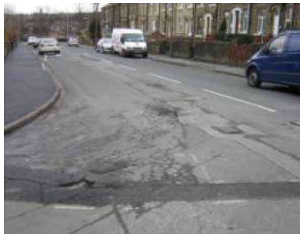
Potholes, image courtesy of David Mazurke
