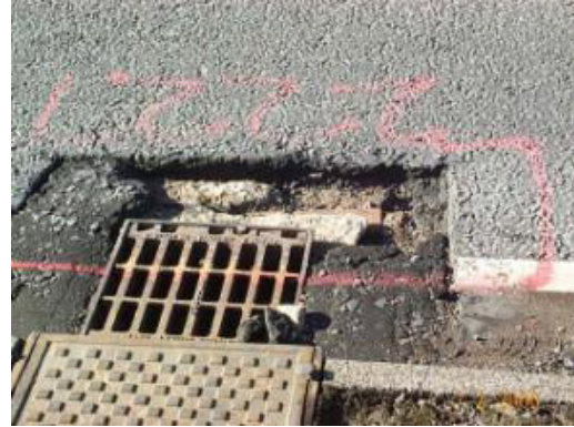
Damage to ironworks, image courtesy of Atkins
